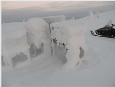
LiDARs and Power supply in operation in January at Olostunturi, Finland
