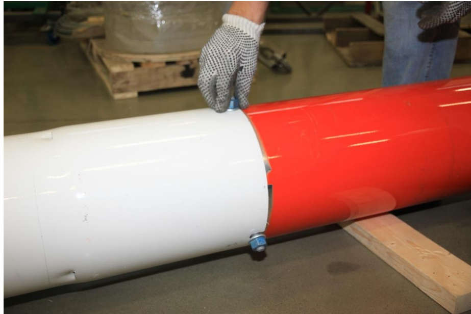
Picture 3-20: Nuts/bolts hand tightened
