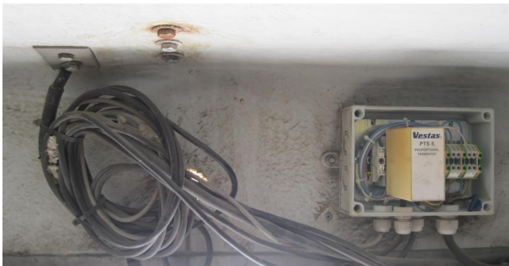
Figure 1 | Junction box for old sensor wires
