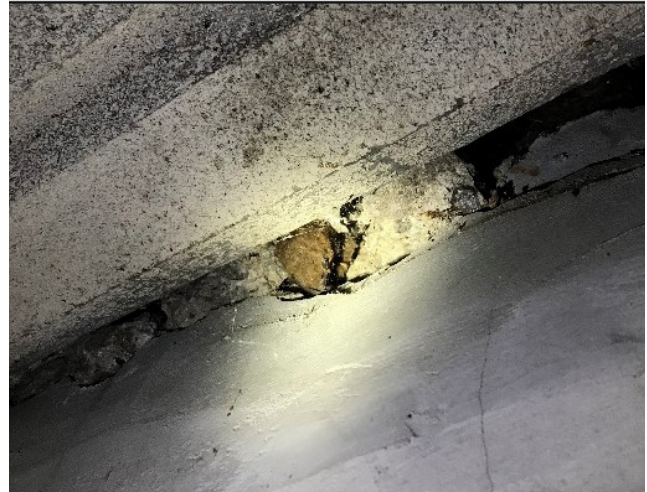
Figure 4. Roosting Bat Trapped in Tar from Road Maintenance
