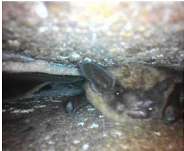
Figure 7. Big Brown Bat Inside of Expansion Joint
